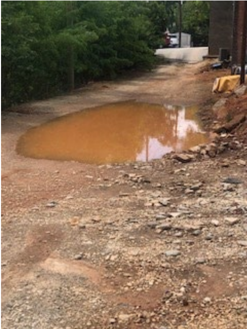
Uncovered drain located behind Steak House.
