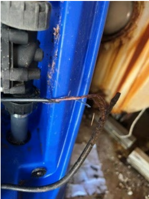
Rewired chlorinator on pool.
