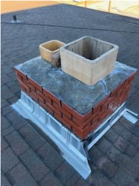
Sealed Police roof. Was leaking.
