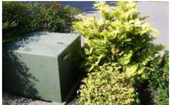
Utility connection screened with plantings
